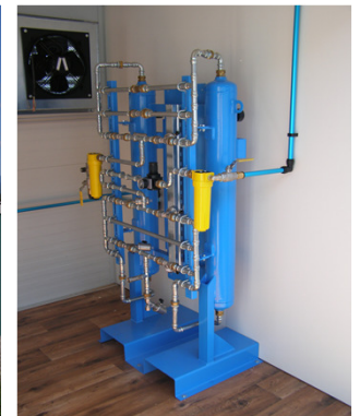
Picture: Micro adsorbent vessels for cleaning and upgrading of raw biogas to biomethane phase
