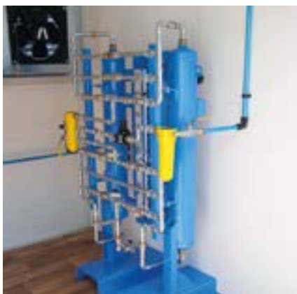
Enota za čiščenje in nadgradnjo bioplina do faze biometana Unit for cleaning and upgrading biogas to the biomethane phase
